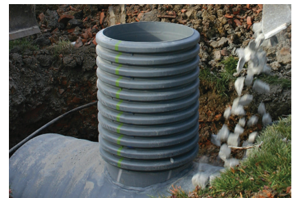
HP Storm Water Harvesting Cistern
