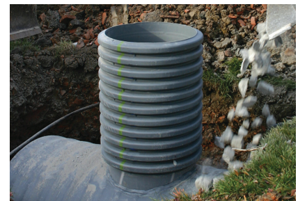
HP Storm Water Harvesting Cistern
