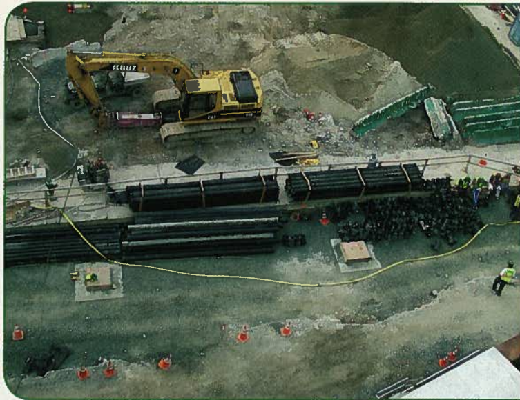
Figure 2: Designed as a grid and installed 85 feet underneath, the drainage system for the 3.5-acre site uses more than 1.5 miles of corrugated HDPE pipe.
