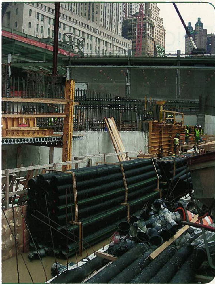
Figure 1: Miles of ADS corrugated HDPE pipe was used to construct the underground water drainage system to help the World Trade Center Memorial project meet LEED certification requirements.
