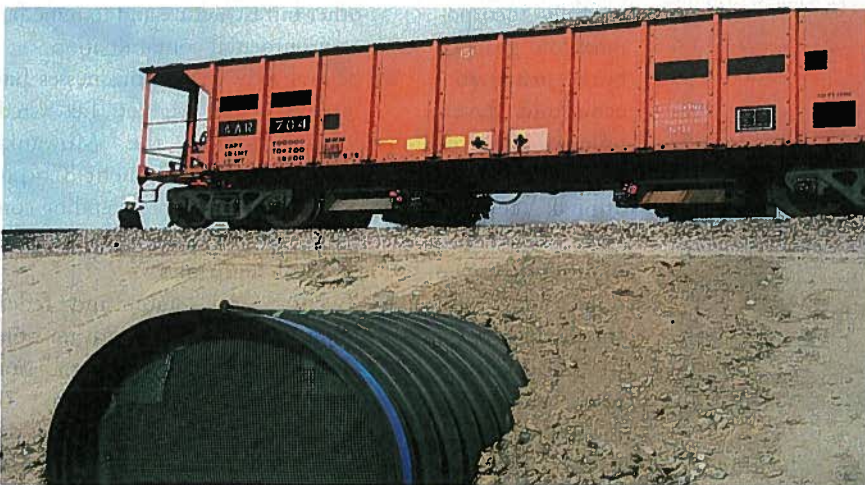
Eighty 315,000-lb rail cars plus four locomotives were repeatedly run over the HDPE pipe with just four ft of cover from the top of the pipe to the bottom of the rail.
