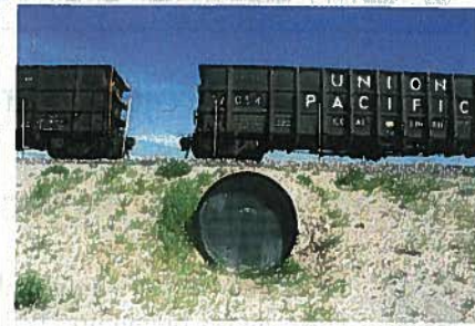
After 96 million gross tons of heavy axle loading, the pipe performed perfectly.
