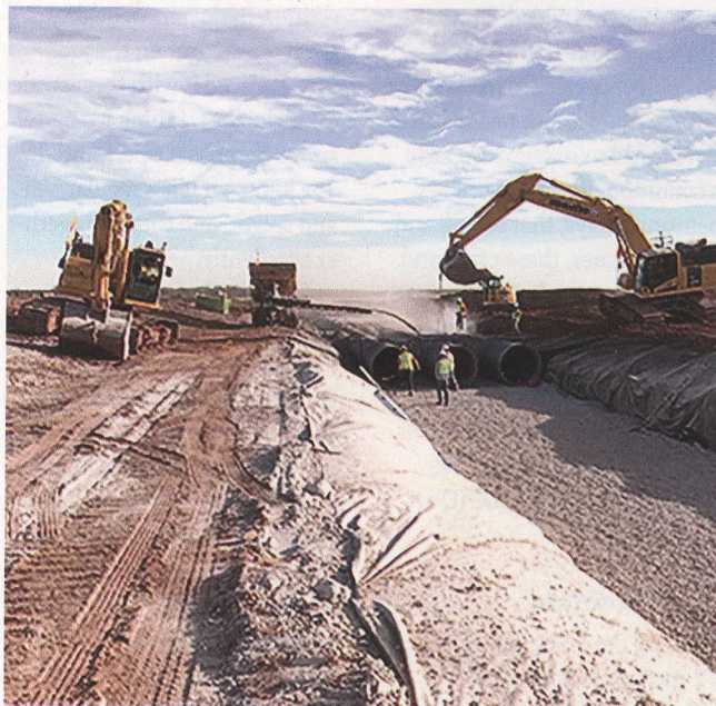
More than 21,000 linear feet of 60-inch-diameter pipe was placed in the 26-foot wide trench to create a French drain to provide drainage between two active U. S. Air Force runways at Sheppard Air Force Base.
