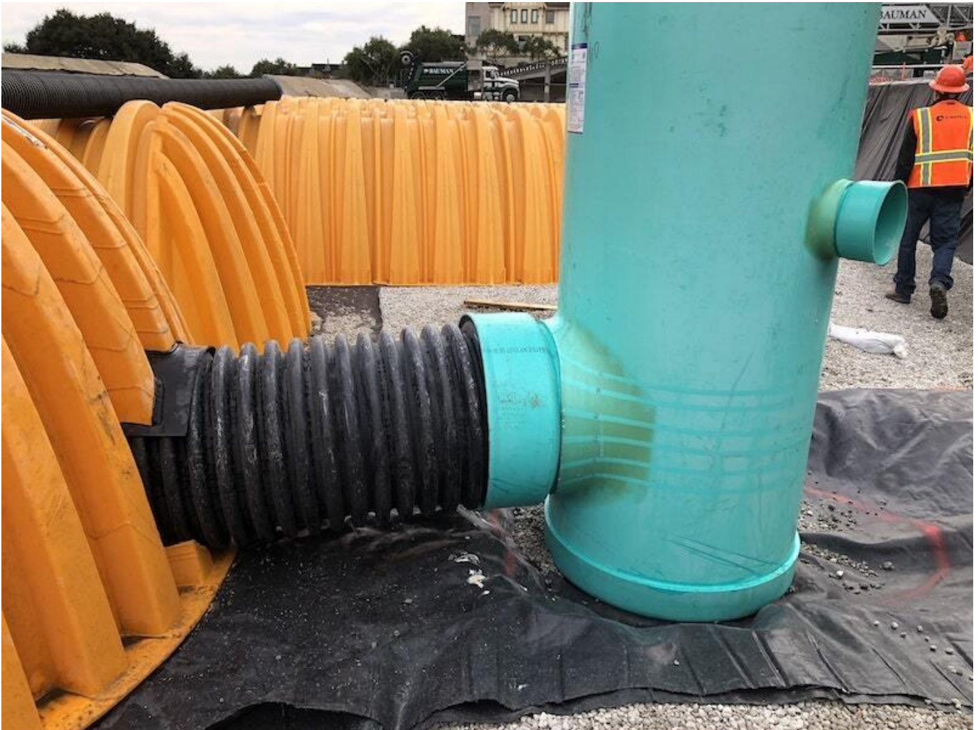
Four 36-inch diameter ADS Nyloplast units with ladders provide access to the system.
