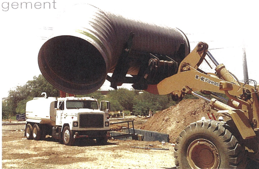
A prefabricated section of N-12 HP pipe is put in place for the road expansion project.
