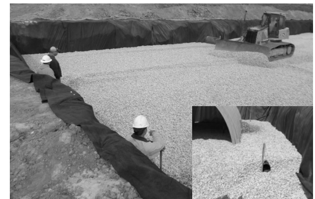
Place clean, crushed, angular stone foundation 150 mm (6") or 100 mm (4") with a single layer of Geogrid BX124GG. See plans for foundation stone design. Compact to achieve a flat surface.
