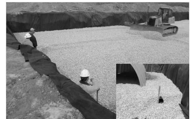
Place clean, crushed, angular stone foundation 150 mm (6") min. Compact to achieve a flat surface.
