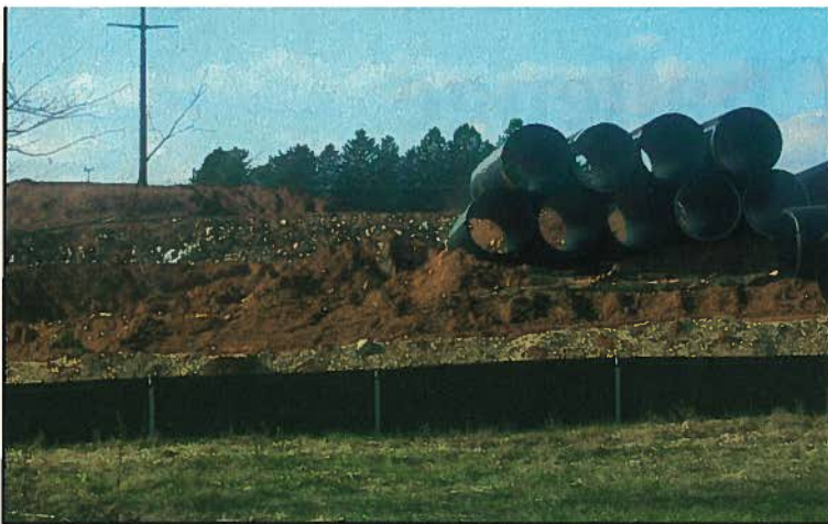
A field of pipe waits to be installed for the new shopping center in Hagerstown, Maryland. More than 6,200 feet of 48-inch diameter corrugated HDPE pipe from ADS was used to construct the storm water detention system.
