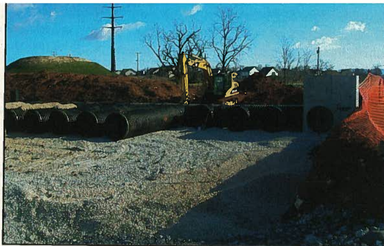
Lateral sections of HDPE pipe are put into place and connected to the storm water detention system's manifold.
