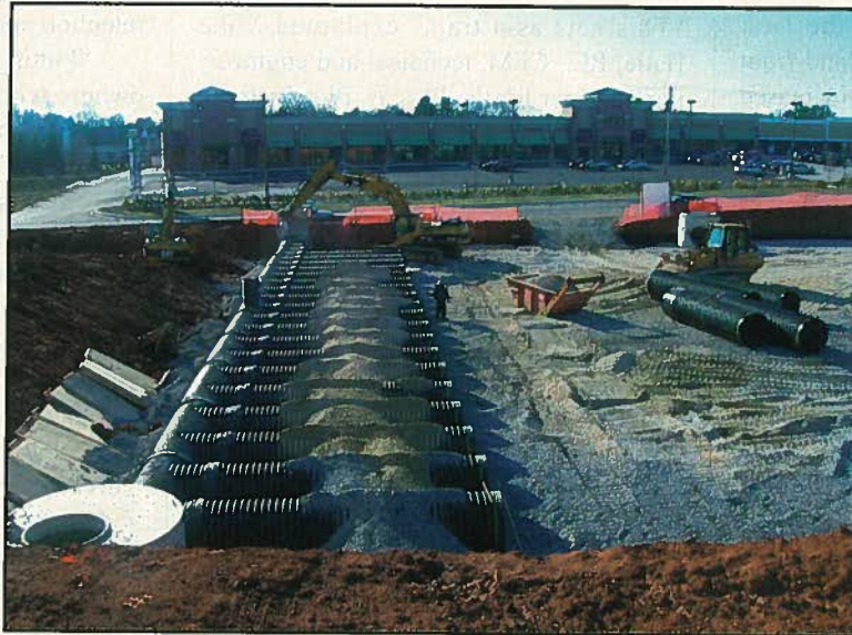
The storm water detention system for a new food store complex was built using 48-inch corrugated HDPE pipe and installed under the parking lot to maximize retail space.
