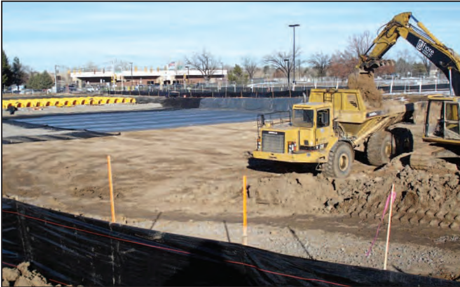
Fiore & Sons nears completion of excavation of Basin 1. Arapahoe Utilities & Infrastructure has already begun installing the rubber membrane liner and placing rock and StormTech chambers, background.
