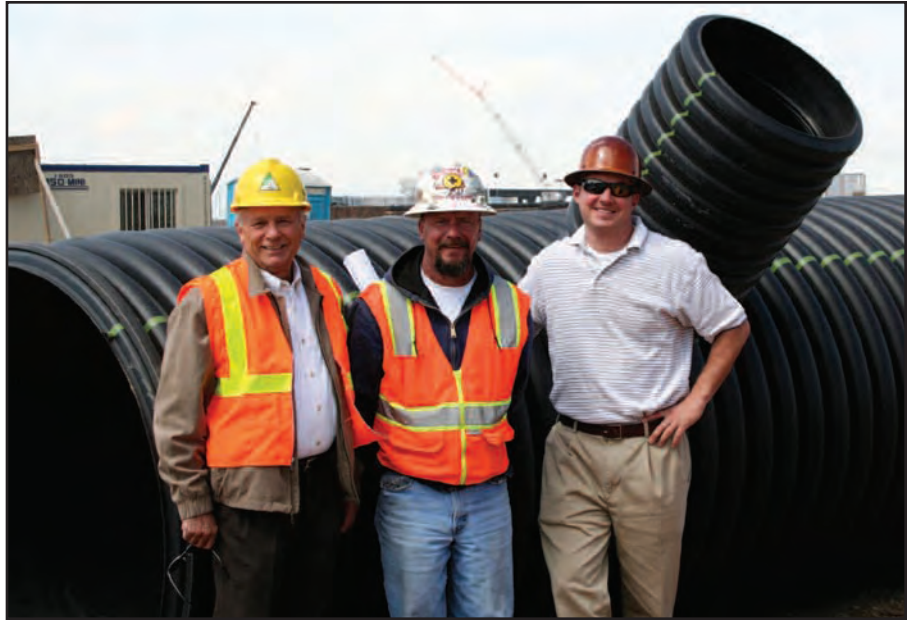
Kael Blair, project supervisor for Arapahoe Utilities & Infrastructure, center, poses with Jim Heintz, left, and Mark Kaelberer of Advanced Drainage Systems beside one of ten ADS water quality units being installed on The Streets At SouthGlenn.
