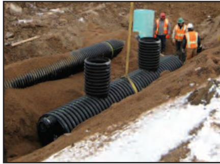
ADS water quality unit is installed in one of the development's subsurface detention basins.
