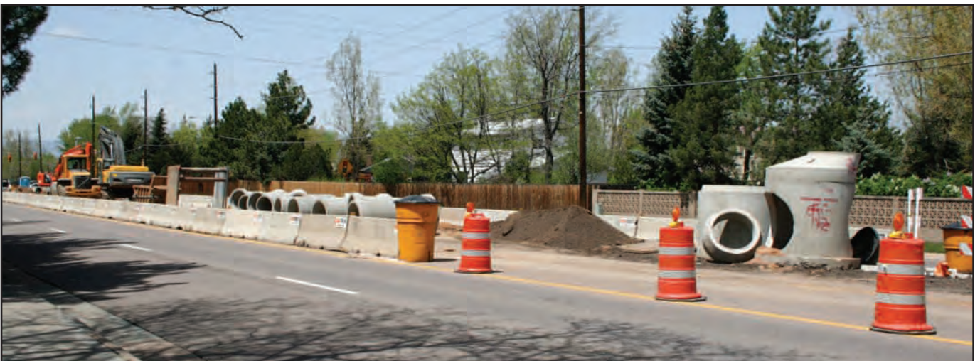
Henderson-based Scott Contracting is upgrading storm sewer under Arapahoe Rd. west of Race St. for City of Centennial.
