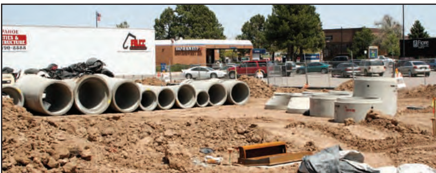
Reinforced concrete pipe and manholes await installation at The Streets At SouthGlenn. Firebaugh Precast supplied the manholes and Rinker Materials supplied the RCP.
