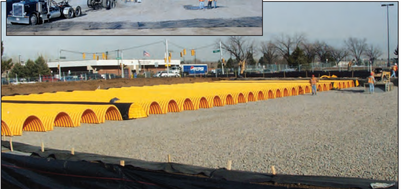
StormTech chambers are placed six inches apart on 2 1/2 feet of 1 1/2-in. rock spread on a nonpermeable rubber liner. Rock is placed and rough graded by wheel loaders and skid steers. Isolator row can be seen wrapped in fabric and with the chamber end cap installed.
