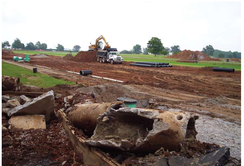
Three runs of perforated pipe were put in, running parallel to each other around the track, spaced 20 feet apart.
