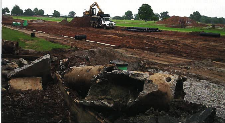
Keeneland Racetrack replaced deteriorating reinforced concrete pipe with high-density polyethylene pipe when it installed a synthetic track surface in 2006.
