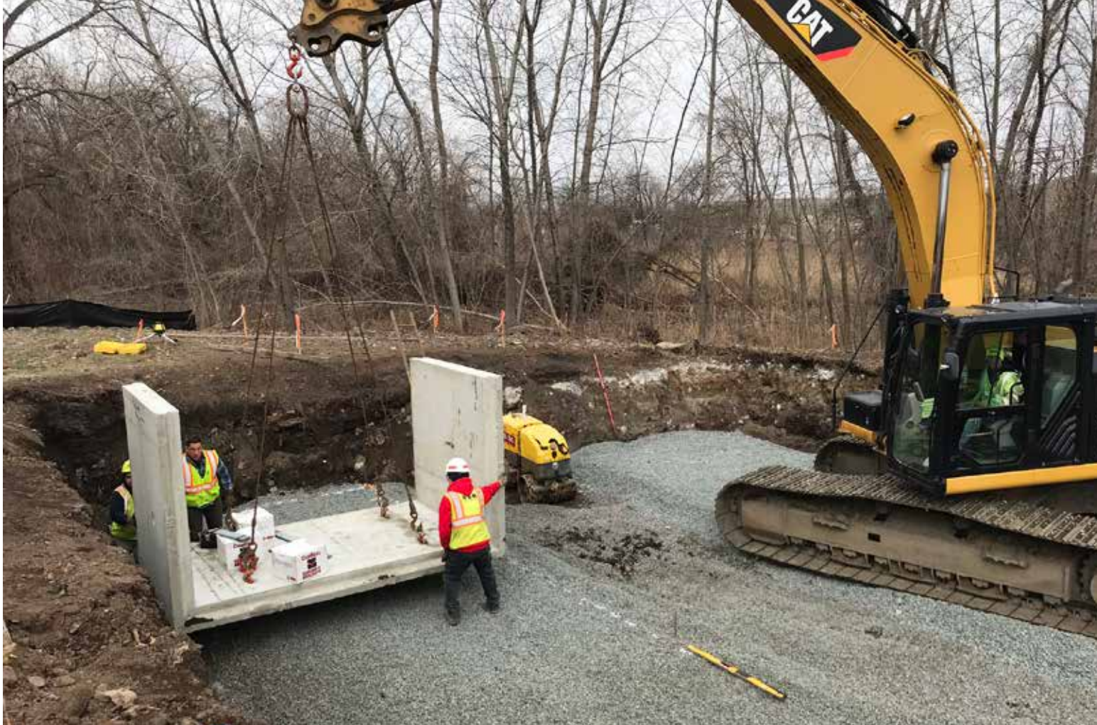
Two concrete vaults were designed and delivered in pieces that could be put in place using an excavator so the contractor would not have to add a crane to the heavy equipment list.
