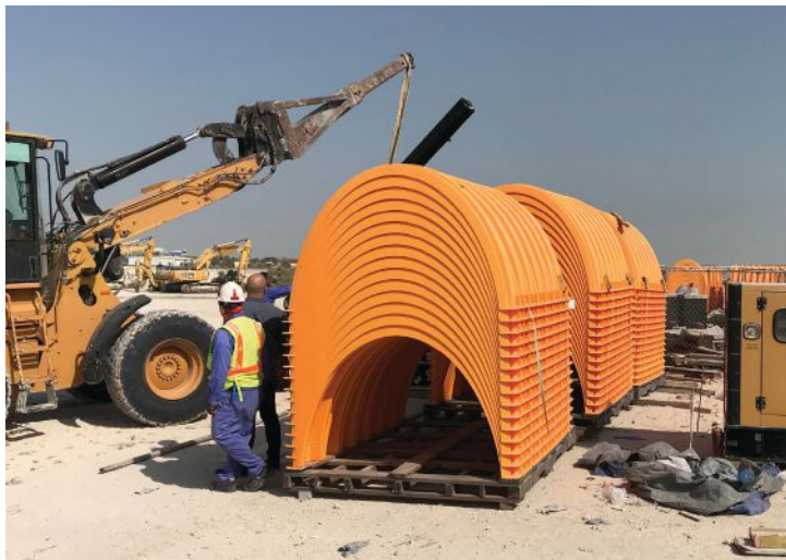
The 7,000-plus StormTech Chambers were delivered on pallets and each one was easily installed by the crew.
