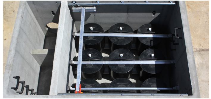
BayFilter Vault Overview
