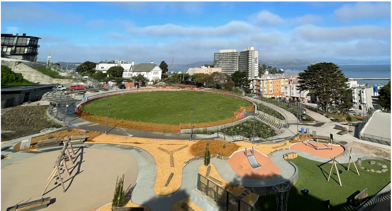
Francisco Park, San Francisco, Ca; (Front cover: StormTech Chambers being installed at Francisco Park).
