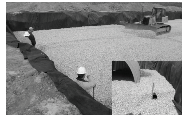
Place clean, crushed, angular stone foundation 6" (150 mm) or 4" (100 mm) with a single layer of Geogrid BX124GG. See plans for foundation stone design. Compact to achieve a flat surface.
