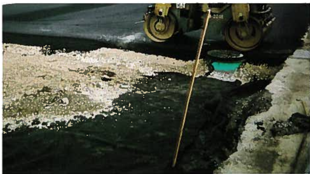
Workers carefully level and compact the final asphalt surface for the auto dealer sales lot around one of the 21 surface drains.
