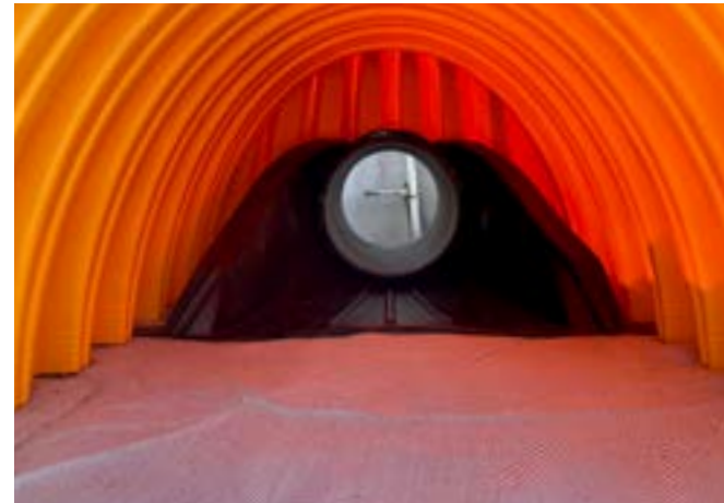
Looking down the Isolator Row PLUS
