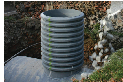
HP Storm Rainwater Harvesting
