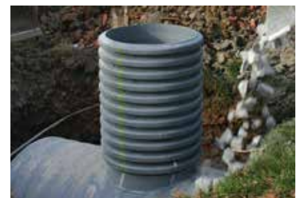
HP Storm Water Harvesting Cistern
