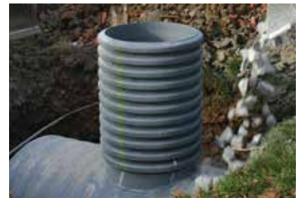
HP Storm Water Harvesting Cistern
