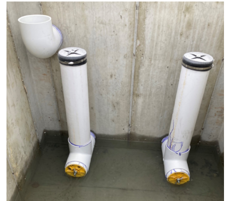
Figure 1: Pipes in pretreatment cell, 2 inlet pipe assemblies and a bypass pipe/elbow
