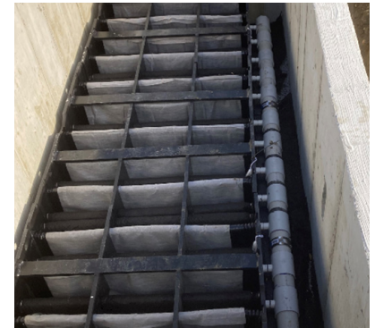
Figure 9: EcoPure Manifolds (3 shown in vault)
