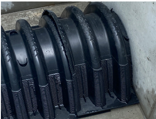
Figure 4: Chamber flush against the wall
