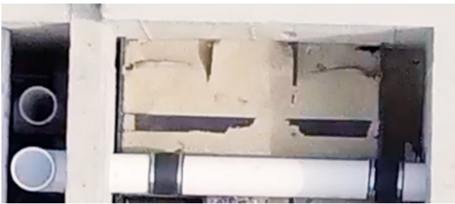
Figure 11: Bypass pipes with Fernco
