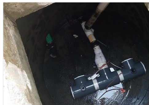
Manifold Tee View of a Cleaned System
