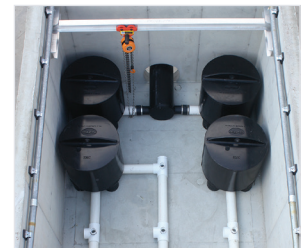
Vault Internal Assembly
