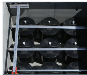
BayFilter Vault Overview
