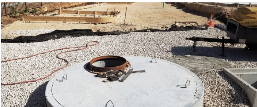
Top: The Natural Grocers site was built and designed with a 100-year storm event in mind and can hold 17,000 gal of storm water.
